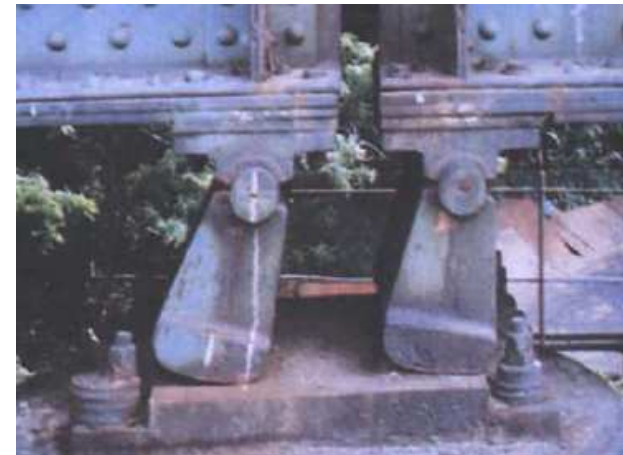
Fonte: BRIDGE INSPECTION MANUAL – NY'S DOT
