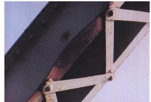
Fonte: BRIDGE INSPECTION MANUAL – NY'S DOT
